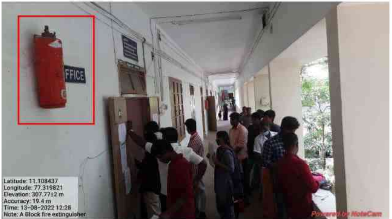
FIRE EXTINGUISHER IN A BLOCK
