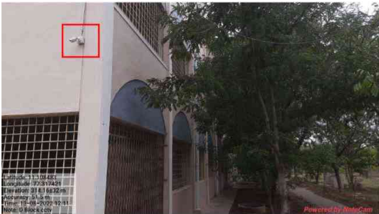
CCTV IN D BLOCK
