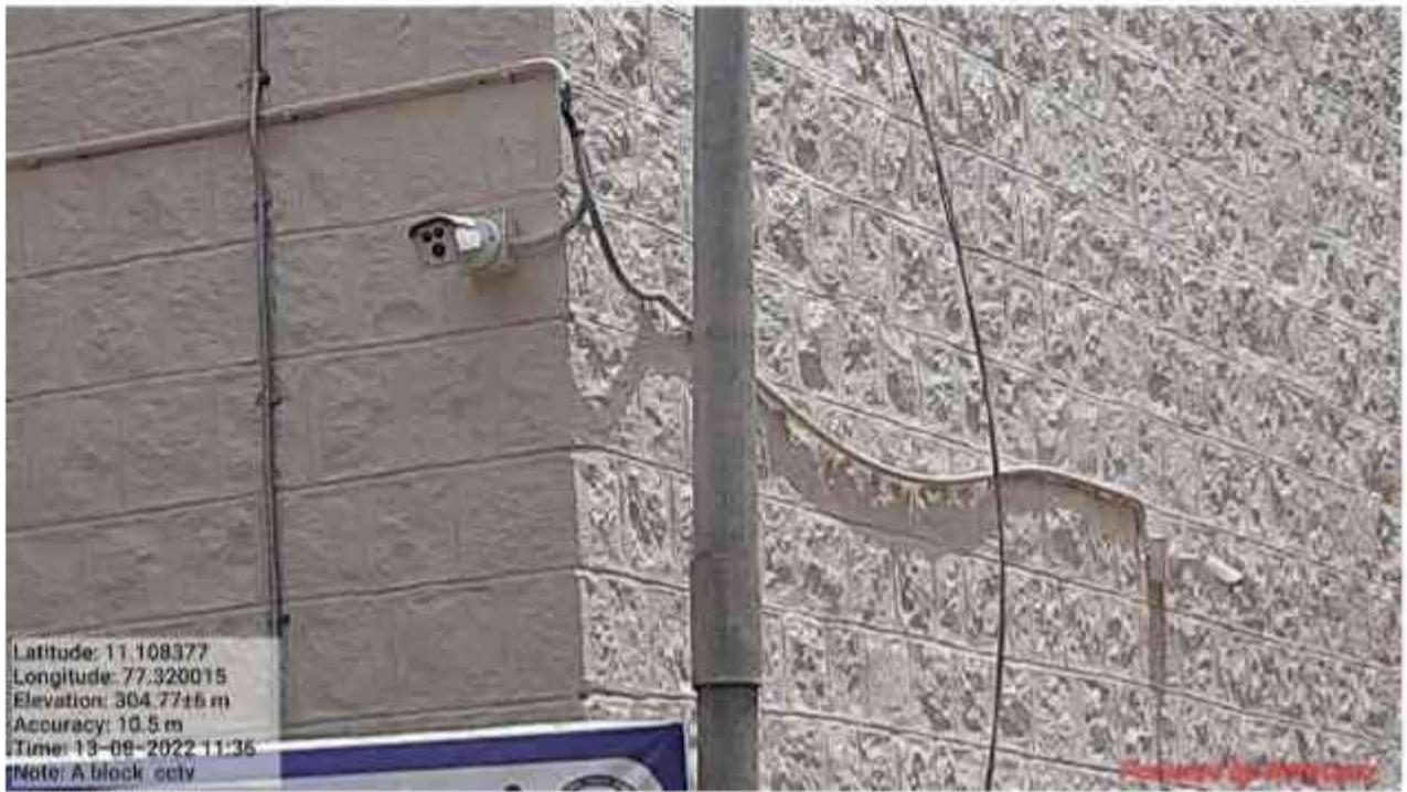
CCTV IN A BLOCK
