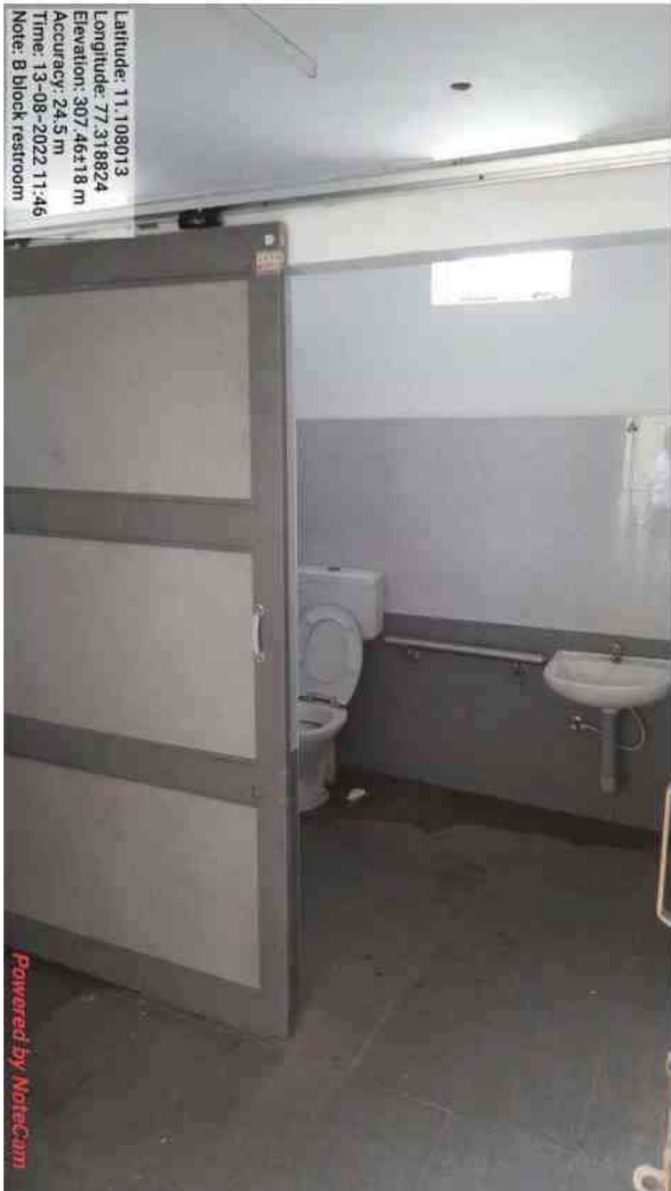
DIVYANGJAN-FRIENDLY RESTROOM IN B BLOCK
