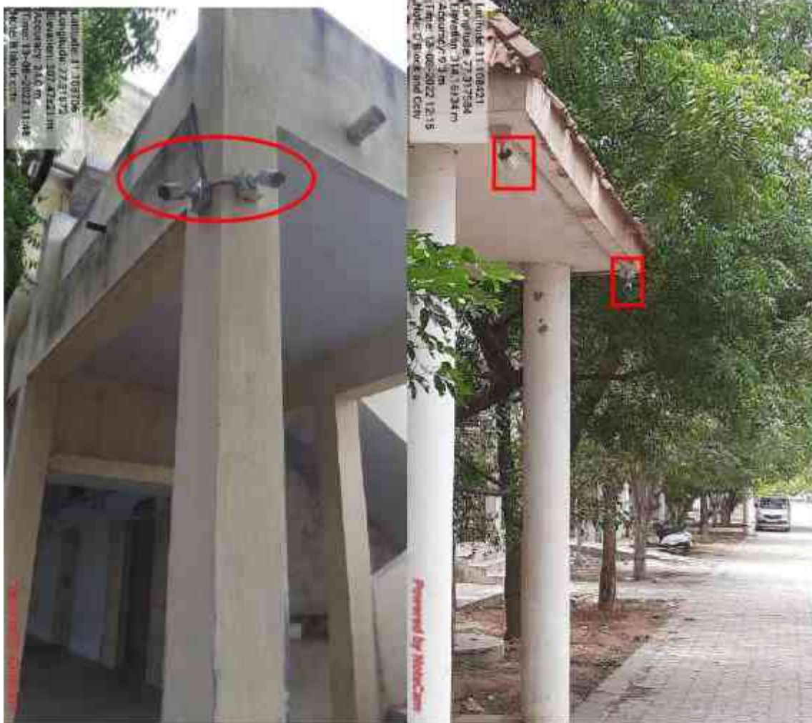
CCTV IN A, B AND C BLOCK
